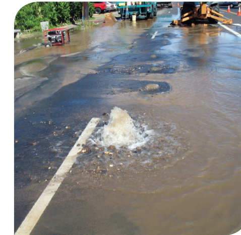
Flooding can make locating and accessing valves difficult
